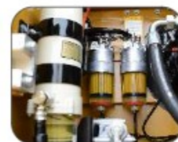
Centralized 3 stage fuel filtration system
