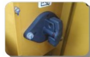
Battery cutoff switch
